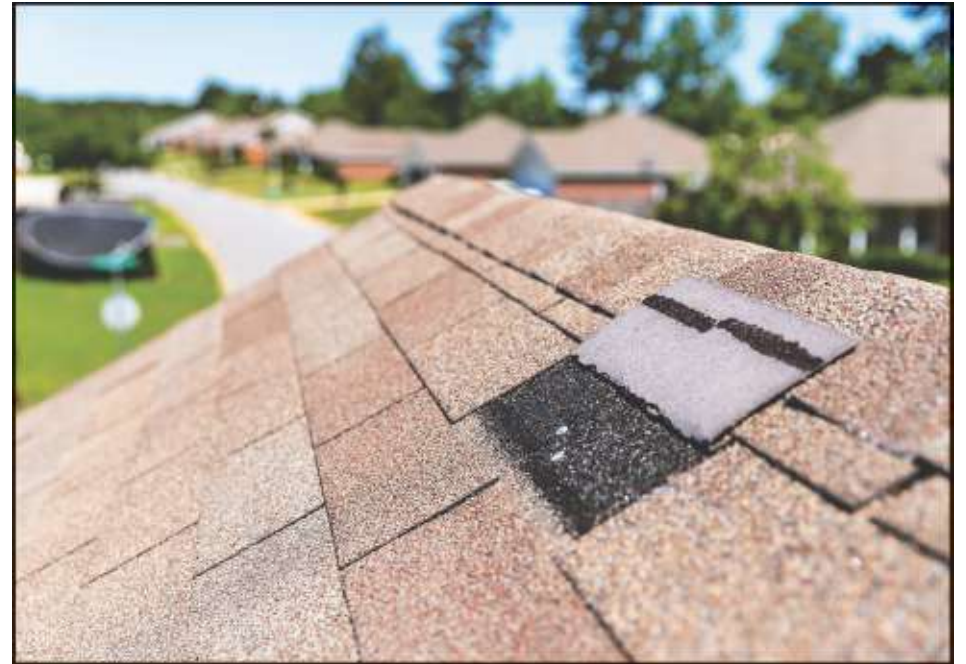
Missing shingles on roof due to storm damage.
